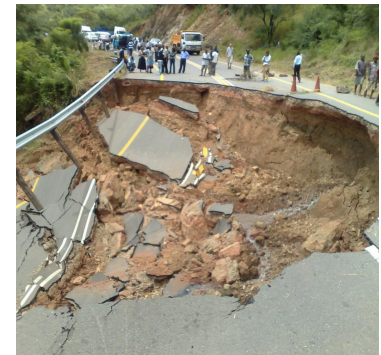
16 Road washed away (Lusaka)
