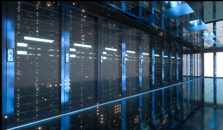
Interxion Data Centers EcoStruxure Power , Building, IT Solutions
