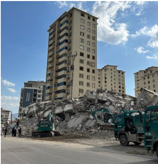
Building in Dogukent, Kahramanmaraş which survived the first event but collapsed in the second earthquake (collapsed building in foreground of photo). (Ref. 7)
