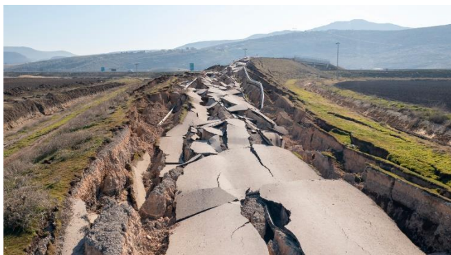
Earthquake damage to a road in Turkey. A new model suggests a period of "aseismic" movement occurs before an earthquake fault ruptures. (Image credit: yasharu/Getty Images)
