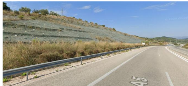
Google Streetview image showing the site of the 2 February 2026 landslide on the Ionian motorway in Greece.
