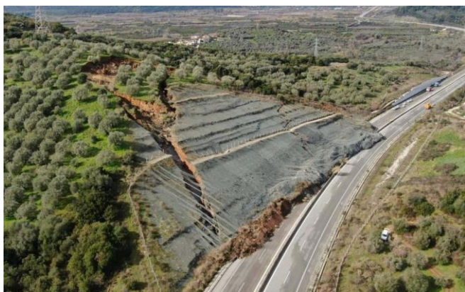
The 2 February 2026 landslide on the Ionian motorway in Greece. Image from ERT via ekathimerini.
